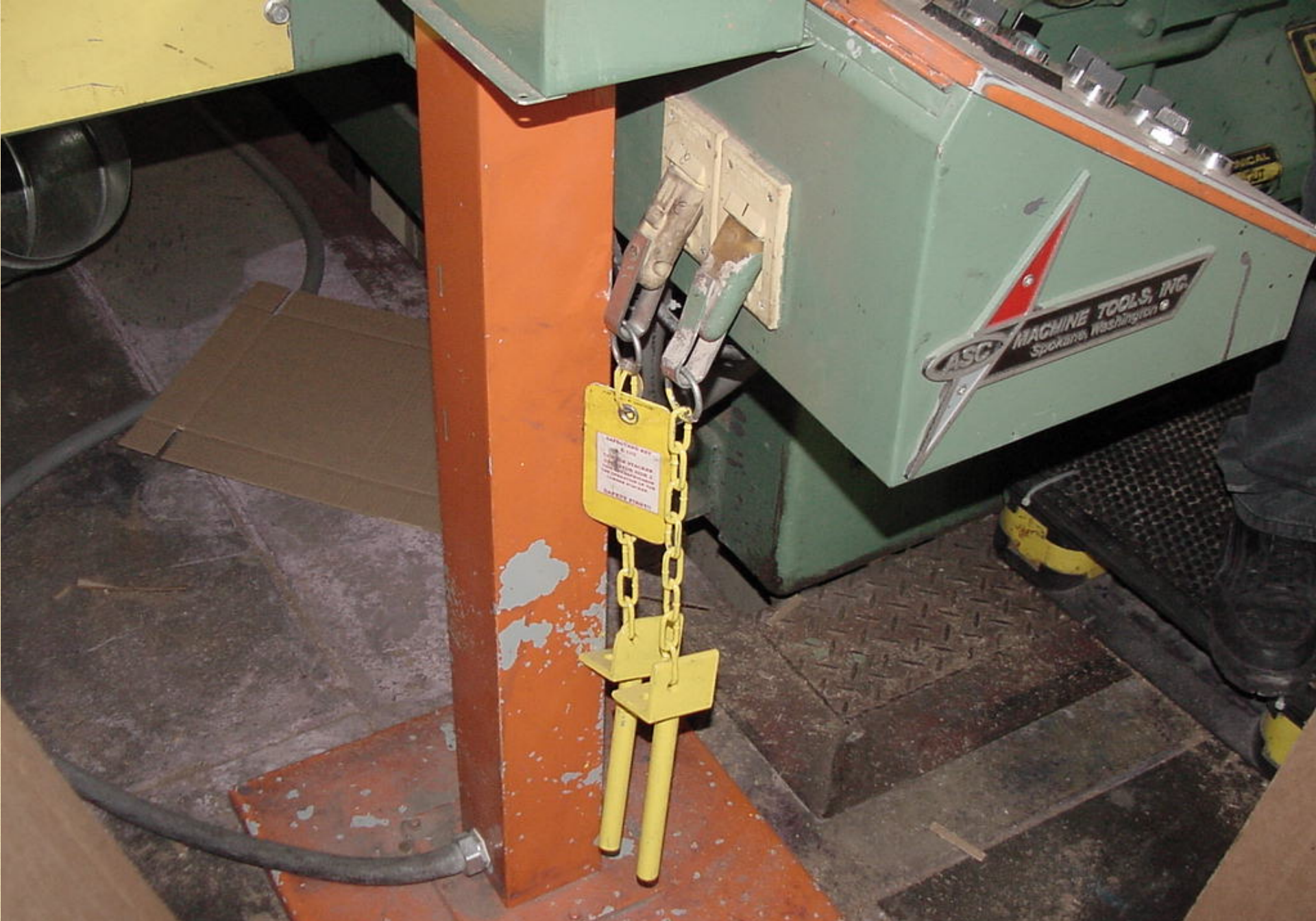
Load Former Disconnects & Safety Pins
